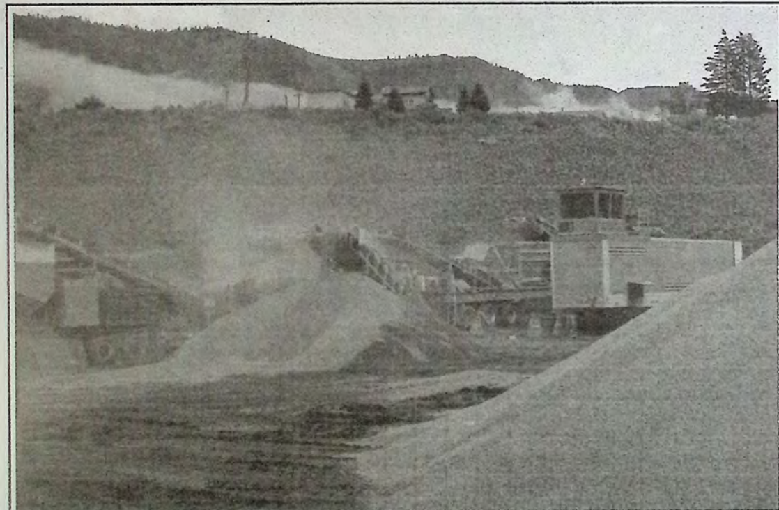
Cantex-Okanagan Construction Ltd. was recently contracted by the Village of Keremeos for a whole lotta' shake, rattle n'roll. Crushing and sorting aggregate may involve putting the material through a screening process more than once. There are five sizes of rock in the aggregate world: boulders are larger than 10 in. (254mm) in diameter; cobbles are 2.5 to 10 in. (64 to 254mm) in diameter; pebbles are .16 to 2.5 in. (4 to 64mm) in diameter; granules are .08 to 0.16 in. (2 to 4mm) in diameter; and grains are .04 to .08 in. (1 to 2mm) in diameter. Did you know that for all its uses, about one truckload of rock is used for each man, woman and child living in BC each year? Photo: Arlene Arlow
