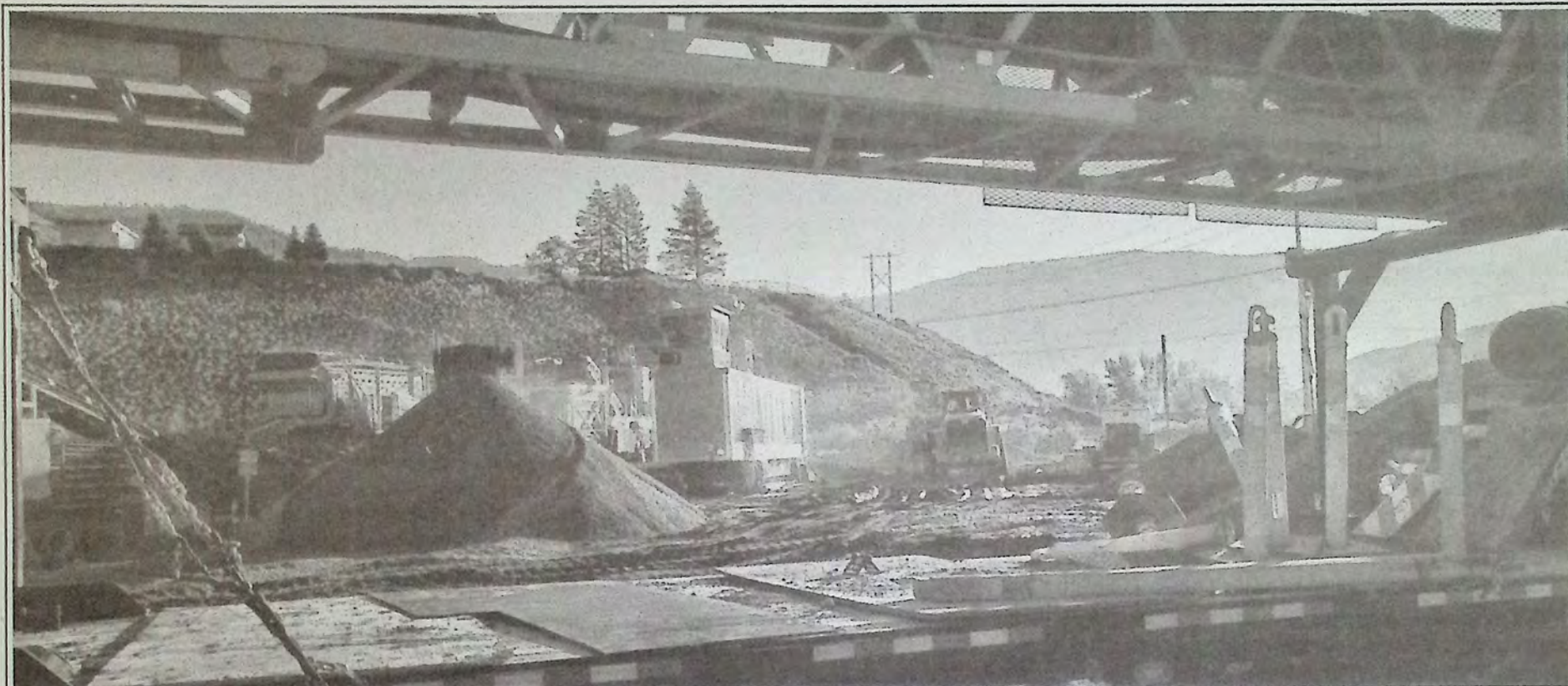
The Village of Keremeos has entered into an agreement with Cantex Okanagan to make winter road sand as well as recycle old concrete and asphalt they have been storing near the Skateboard Park. According to Public Works Foreman Jordy Bosscha, "This will stockpile at least five plus years of road sand that we will not have to buy in the winter and also provide crushed road base that can be spread to upgrade non-paved roads in the Village." Before crushing old concrete, all metal and rebar must be removed from the concrete. The concrete is broken into approximately one-foot chunks before processing. Paul Carey, General Manager of Cantex commented, "When crushing concrete we may end up applying magnets to the concrete before and during processing to remove wayward metals. Metals wreak havoc on crushers." Photo: Marty Menzies
