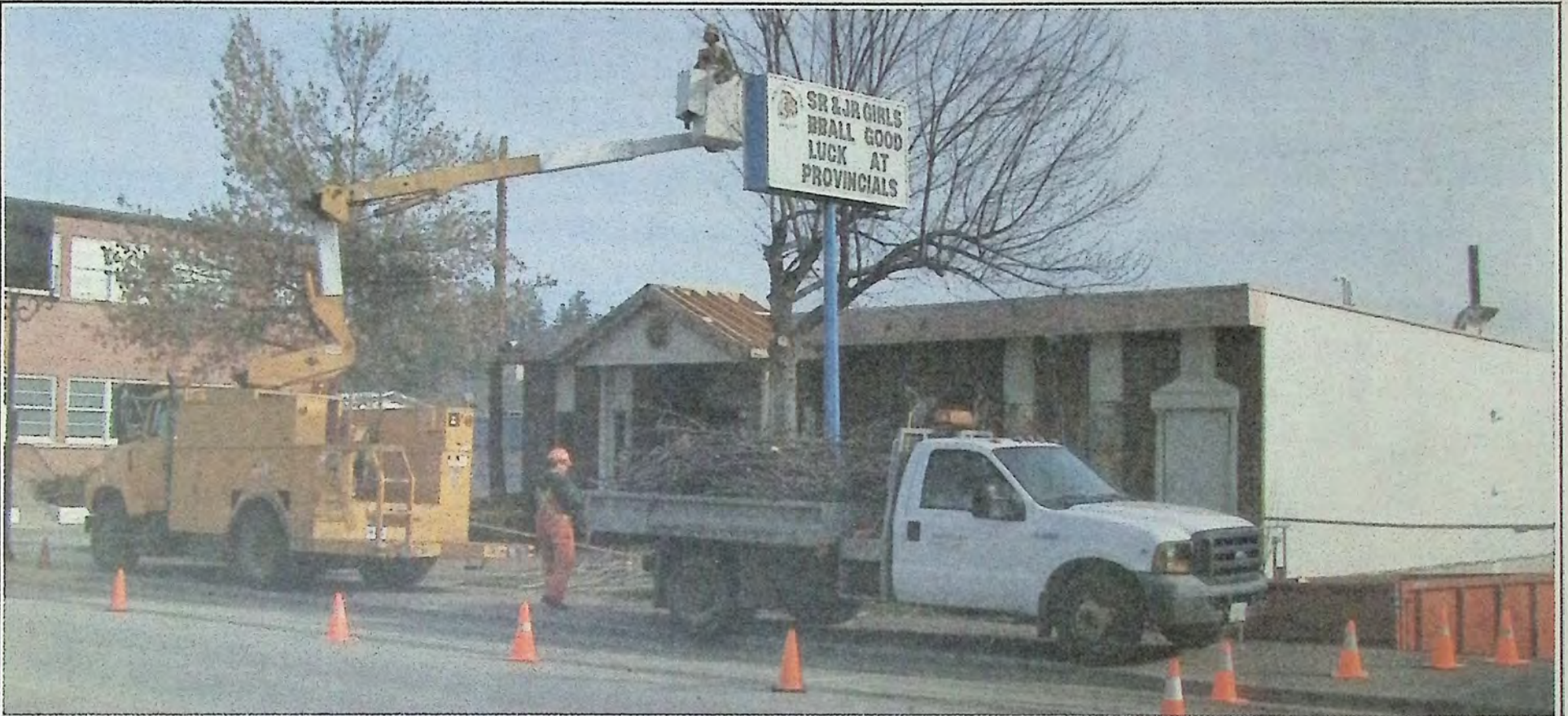
One of the biggest changes to downtown Princeton in 2015 was the renovation of the former town hall building into a tourist information centre. What will change in 2016? *
