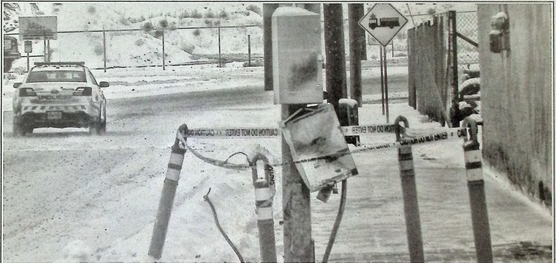
Constant snowfalls and freezing conditions made for a number of road accidents. Just one of the many victims was the control box at the corner of 7th Avenue and 7th Street in Keremeos which was damaged early last week. Photo: Marty Menzies
