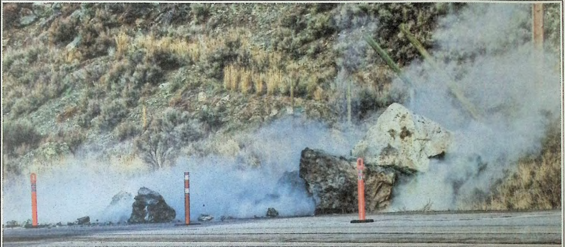
Calling the blast 'anti-climactic', News Leader photographer Marty Menzies was on hand February 2nd when highways crews took care of the boulder that had been sitting along Highway 3 west of the Red Bridge at Keremeos. The rock had rolled down the hillside almost two week before. Photo: Marty Menzies
