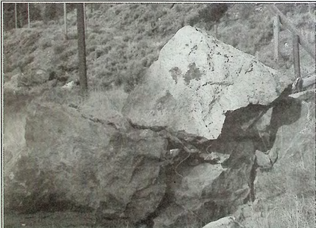
Sometimes you have to blast a rock into smaller pieces before you can haul it away. That was the case February 2nd at a location along Highway 3 just west of the Red Bridge. Photo: Marty Menzies
