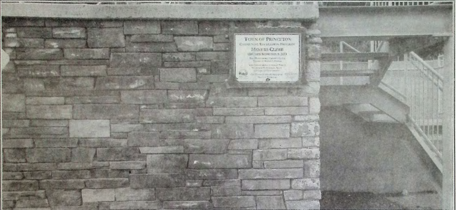
Have you noticed what's happening to the wall at the bottom of Miner's Climb? It's crumbling away as can be seen on the plaque side of the structure which is also discoloured. Photo: Brenda Engel
