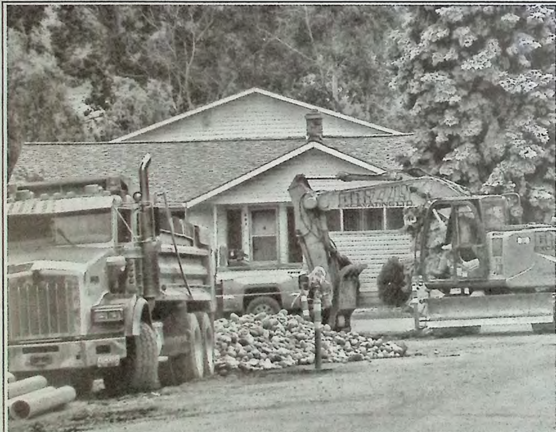
The repaving and upgrade to 4th Street between 11th Avenue and 12th Avenue started last Thursday (May 18) and will level out the blacktop that's been breaking up on that stretch for some time. Photo: Marty Menzies
